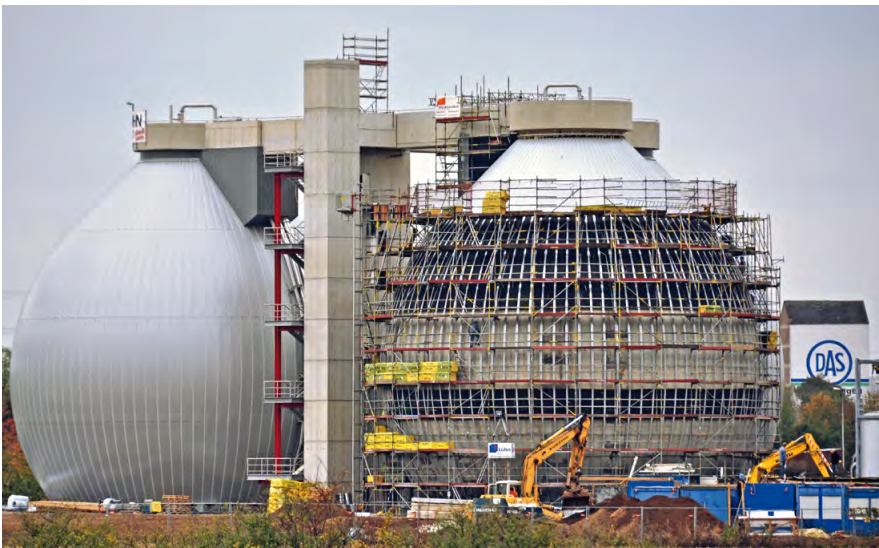
Sewage Plant, Dueren, Germany
