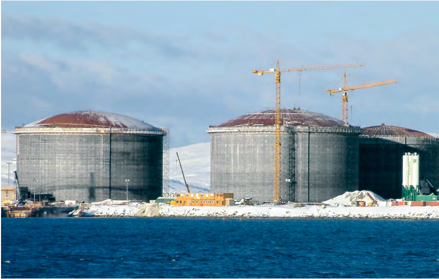
LNG Tanks, Snøhvit project, Melkøya Island, Norway
