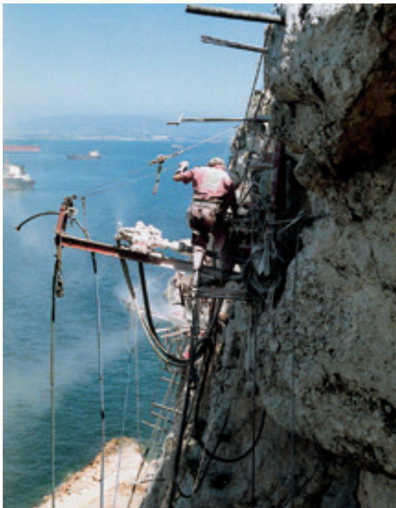
Slope stabilization using DYWI® Drill Hollow Bar Anchors at the Rock of Gibraltar
