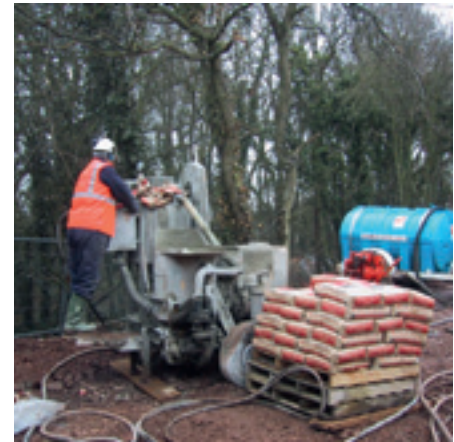
Grout pump with colloidal mixing unit
