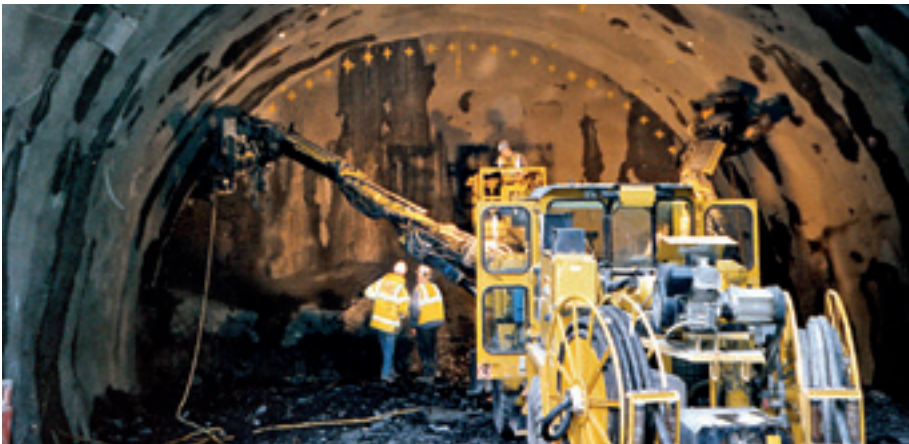
DYWI® Drill hollow bar spiles for the stabilization of a launch adit for a TBM
