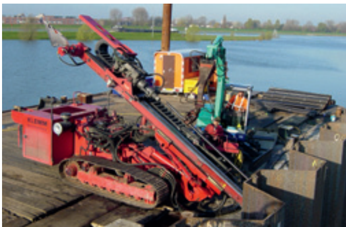
Hollow bar drilling from a floating barge for sheet pile tie back
